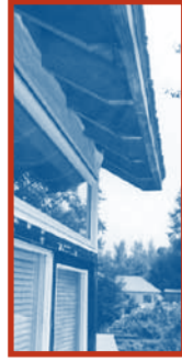
Open eaves, vents not screened (6 pts)
